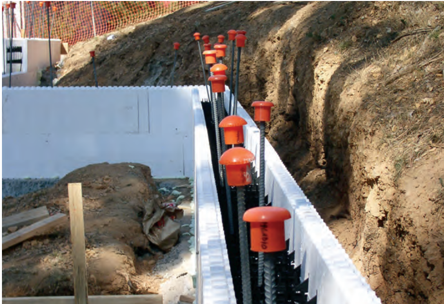
Figure 6.7 – Plastic mushroom caps on protruding steel bars
